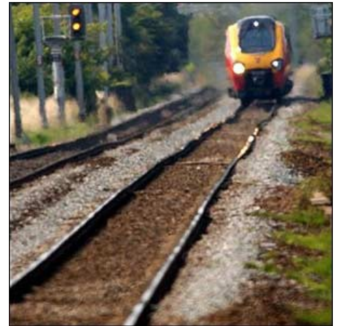
Soaring temperatures in the summer of 2003 forced rail networks to be closed because the track buckled in the heat. (Courtesy BBC).
